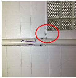
Support strap(s) are deteriorated/detached for plumbing drain waste pipes.
