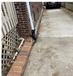
There are no splash blocks installed on some of the gutter downspouts for the roof drainage system for the Roof of the Home.
