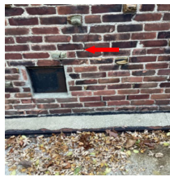
There is an area of cracking in the exterior brick wall cladding.
