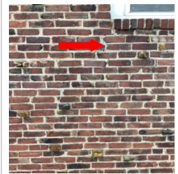
There is an area of cracking in the exterior brick wall cladding.
