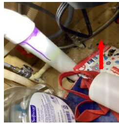
Under the sink in the kitchen, there appears to be an active water issue causing some water damage. Further Evaluation is Needed to help prevent more issues, recommend a certified plumber to repair all that is necessary.
