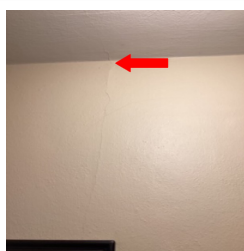
There is a crack in the ceiling working it's way up from the wall in the Hallway.
