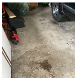
There is what appears to be a typical crack in the concrete slab/floor in the Detached Garage.
