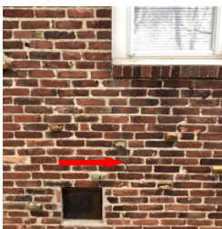
There is an area of cracking in the exterior brick wall cladding.
