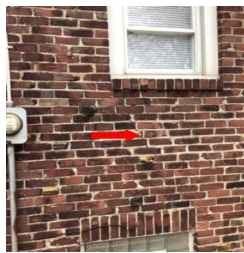
There is an area of cracking in the exterior brick wall cladding.
