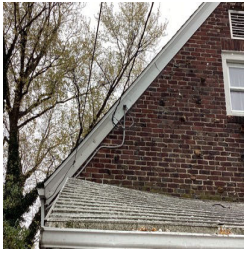
Electrical Service Entry
