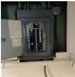
Main Electrical Panel Board Enclosure in the
