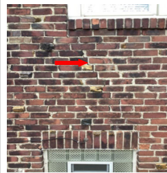
There is an area of cracking in the exterior brick wall cladding.
