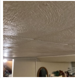
There is sagging in the ceiling in the Bedroom at the Top of the Stairs.
