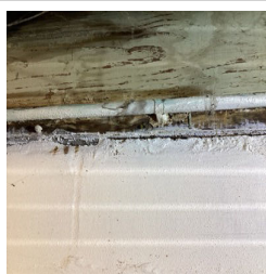
There is a moisture stain on a sill plate in the Basement.
