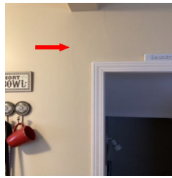
There is a crack in a wall in the Kitchen.
