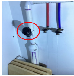
A plumbing drain waste vent pipe has an improper connection in the crawlspace. Electrical tape was used as a cap, with a clamp around it.
