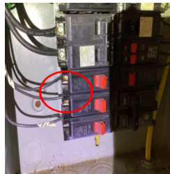
There is corrosion on a circuit breaker in the Main Electrical Panel Board Enclosure in the.
