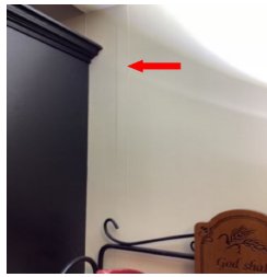
There is detached drywall seam tape on an interior wall(s) in the Kitchen.
