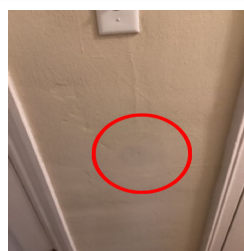
There is an area of noticeable repair to an interior wall in the Hallway.
