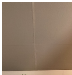
There is what appears to be a typical crack in an interior wall in the Bedroom at the Top of the Stairs.
