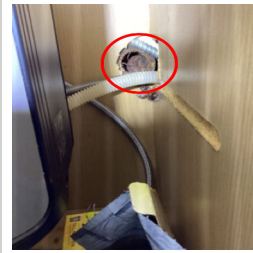
Under the sink in the kitchen there appears to be an open pipe, recommend a certified plumber to repair all that is necessary.
