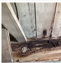
There are areas of fungal growth on wood surfaces in the Basement.
