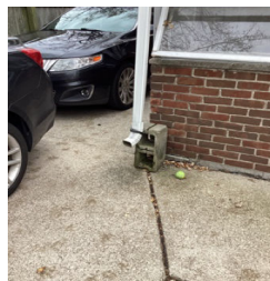
There are no splash blocks installed on some of the gutter downspouts for the roof drainage system for the Roof of the Home.
