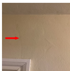
There is an area of noticeable repair to an interior wall in the Hallway.
