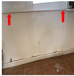
Plumbing drain waste pipes are improperly sloped in the basement. On the left of this picture is going to the main sewer connection, and on the left of this picture is the sump pump is.
