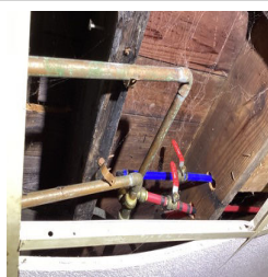
There are damaged floor joists in the Basement.
