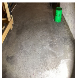
There is what appears to be a typical crack in the concrete slab/floor in the Basement.
