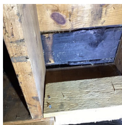
There are areas of deteriorated sub-floor in the Basement.
