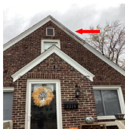
There is an area of missing metal wrap on the fascia on the exterior of the home.
