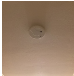
Smoke alarm in hallway
