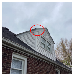
There is an area of detached metal wrap on the fascia on the exterior of the home.
