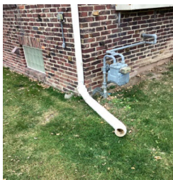
There are no splash blocks installed on some of the gutter downspouts for the roof drainage system for the Roof of the Home.
