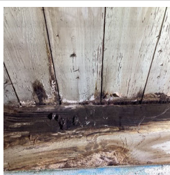
There are areas of fungal growth on wood surfaces in the Basement.
