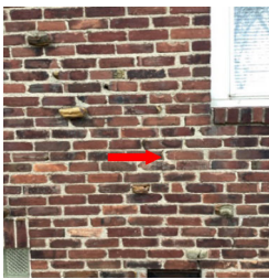
There is an area of cracking in the exterior brick wall cladding.
