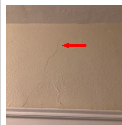
There is a crack in a wall in the Hallway.
