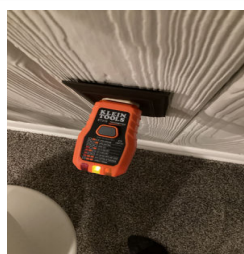
An electrical outlet has an open ground in the Living Room.
