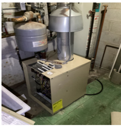
Boiler Heating System
