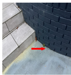
There are cracks that appear to be typical in an exterior service walk.
