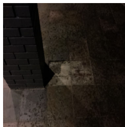
There are missing tile on the exterior Patio(s).
