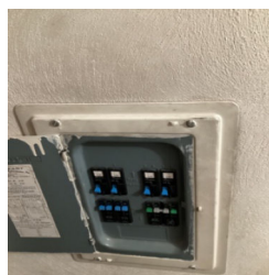
Sub-Electrical Panel Board Enclosure in the closet upstairs off the hallway.
