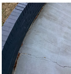
There are cracks that appear to be typical in an exterior service walk.
