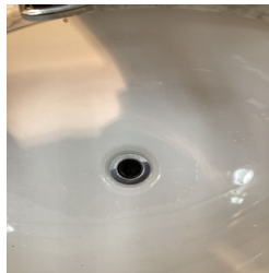
A stopper valve is missing on a sink in the Full Bathroom off the Hallway.
