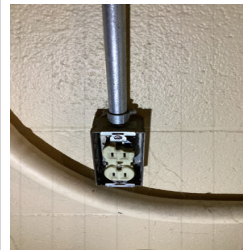
There is a damaged electrical outlet in the Rec Room.
