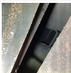
The flue and damper in the fireplace in the wet bar room.
