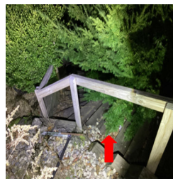
There is no balusters on the steps on the retaining wall.
