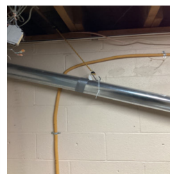
Improper dryer duct installation in the laundry room.
