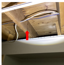
There is an area of staining on the ceiling in the Laundry Room.
