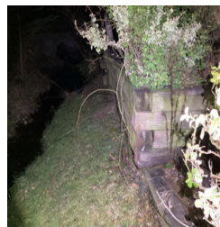
An exterior retaining wall appears to be leaning.
