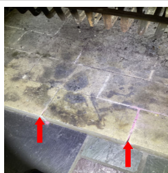
There are crack(s) in the firebox of the Fireplace in the wet bar room.
