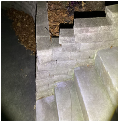
Retaining wall Detaching from the steps.
