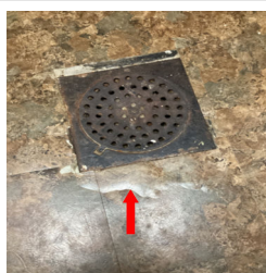
There is an area of soft flooring in the Laundry Room.
