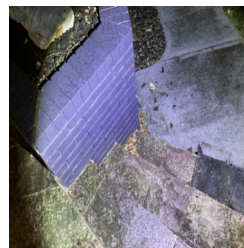
There are cracks in the exterior Patio(s).
