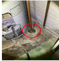
The temperature pressure relief valve is leaking on the Gas Water Heater in the.
