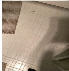
There are cracked floor tiles in the Master Bathroom.
