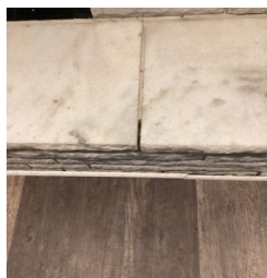
There are cracks in the hearth extension for the Fireplace in the Formal Living Room.
