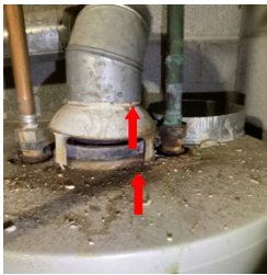
Rust found on the top of the water heater and on the exhaust pipe.
