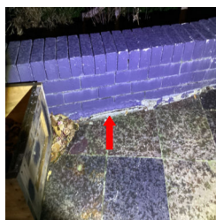
There is a crack in a foundation wall for the raised Patio.
