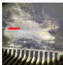
There are crack(s) in the firebox of the Fireplace in the wet bar room.
