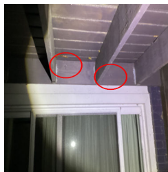
Bolts are improperly spaced on the Components visible on Exterior at the deck.
