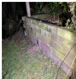
There is an area of deterioration in an exterior retaining wall.
