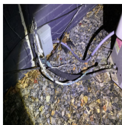
Corrosion found on the cooling unit outside
