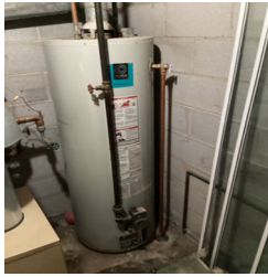
Gas Water Heater in the
