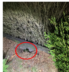
There is a dugout area near an exterior retaining wall.
