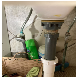
A sink water supply line is corroded in the Full Bathroom off the Hallway.
