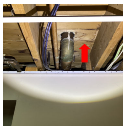
There is an area of staining on the ceiling in the Laundry Room.
