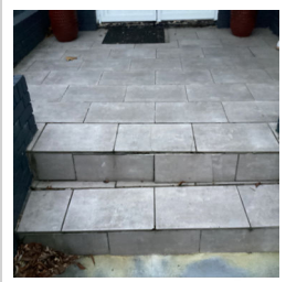
There are cracked and loose tiles on the steps on the service walk, leading into the front door.
