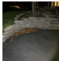
Retaining Wall off the driveway going into the front of the home
