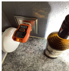
An electrical outlet has an open ground in the Dining Room.
