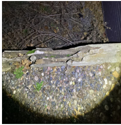
There is an area of damage in an exterior retaining wall.
