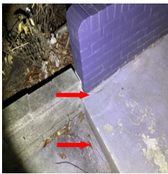
There are cracks in an exterior service walk.
