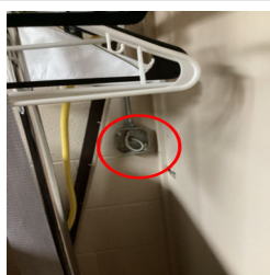
There is an open junction box in the Laundry Room.
