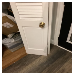
A closet door drags on flooring in the Foyer.
