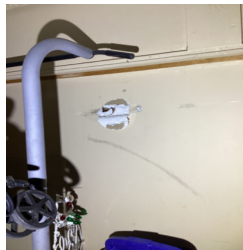
There is a hole in an interior wall in the Rec Room.
