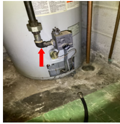
There is no sediment trap/drip leg installed on the gas line for the Gas Water Heater in the.
