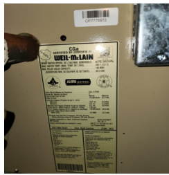
Boiler Heating System Tag
