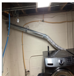
The dryer vent is improper on the interior of the home for the dryer in the Laundry Room.
