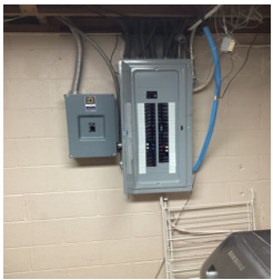
Main Electrical Panel Board Enclosure in the
