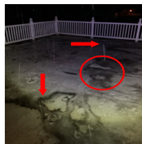
Ponding on the patio floor outside of the master bedroom.
