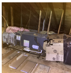
There are makeshift repairs to ductwork in the crawlspace.
