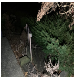
There is an area of damage in an exterior retaining wall steps with vegetation in the way of the steps.
