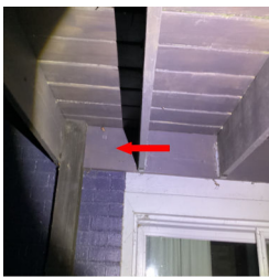
Bolts are improperly spaced on the Components visible on Exterior at the deck.
