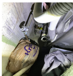
Washer Plumbing/Dryer Venting
