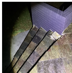
There are cracked, loose and missing tiles on the exterior Patio(s).
