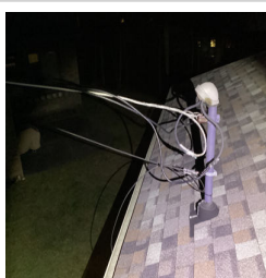
Electrical Service Entry
