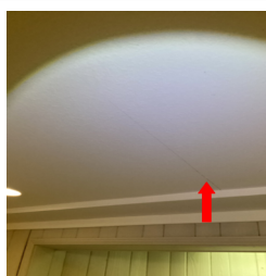
There is a crack in the ceiling in the Living Room.
