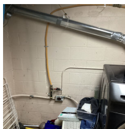
The gas line is improper for the dryer in the Laundry Room.
