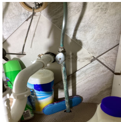
A sink water supply line is corroded in the Full Bathroom off the Hallway.
