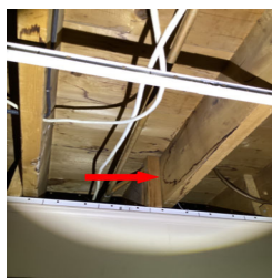
There is an area of staining on the ceiling in the Laundry Room.
