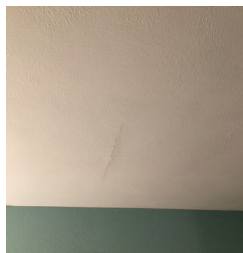
There is what appears to be a typical crack in the ceiling in the Bedroom at the top of the stairs to the right off to the right.
