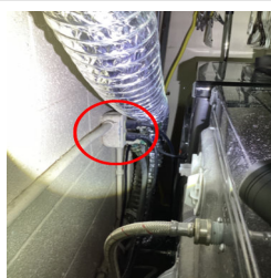
There is no GFCI protection on an electrical outlet in the Laundry Room.
