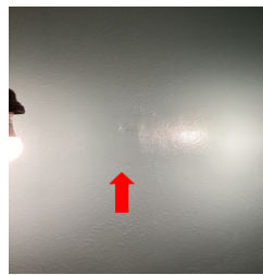
There is an area of noticeable repair to an interior wall in the Bedroom at the top of the stairs to the right off to the right.
