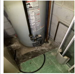
The Gas Water Heater in the is concealed on the interior of the home and is not installed in a proper drain pan with a drain to the exterior.
