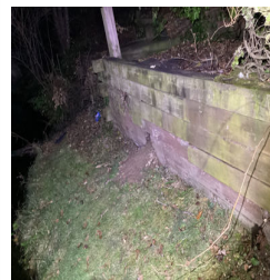
There is a hole in an exterior retaining wall.
