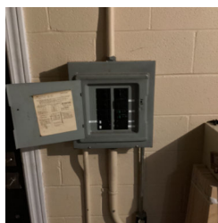
Sub-Electrical Panel Board Enclosure in the rec room.
