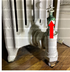
Living Room Radiator
