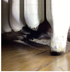
There are moisture stains on the floor in the Living Room.
