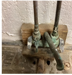
Sink water supply lines are corroded in the Laundry Area.
