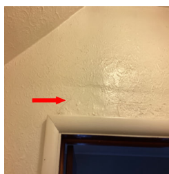
There is what appears to be a typical crack in an interior wall in the Closet between kitchen and living room.
