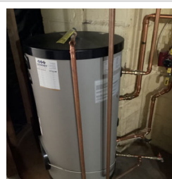
Boiler Heating System
