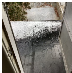
A railing is missing on the Balcony.
