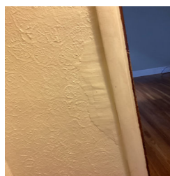
There is an area of noticeable repair to an interior wall in the Closet between kitchen and living room.
