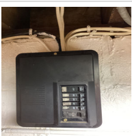
Sub-Electrical Panel Board Enclosure in the
