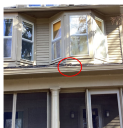
There is debris in the gutters on the Roof of the Home.
