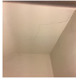
Office closet appears to have a crack on the ceiling, recommend a qualified contractor to repair all that is necessary.
