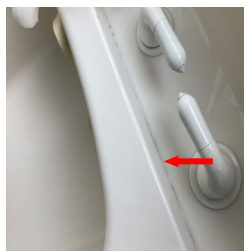
Grout/caulking is deteriorated near the whirlpool/jet tub in the Master Bathroom.
