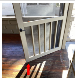
A door drags on flooring on the Front Porch.
