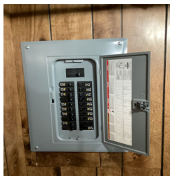
Main Electrical Panel Board Enclosure in the
