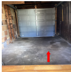
There is what appears to be a typical crack in the concrete slab/floor in the Garage.
