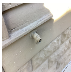
A hose faucet is not operational on the exterior of the home.
