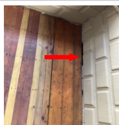
There is a crack in the floor on the Front Porch.
