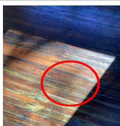
There is bounce in the Front Porch flooring when it is walked on.
