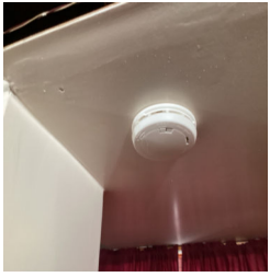
Smoke and Carbon Monoxide Alarm(s) in basement
