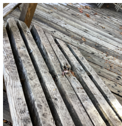
There is deterioration in decking boards on the Deck.
