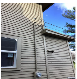
Electrical Service Entry
