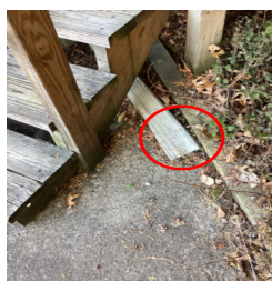
Crushed downspout under the back deck steps.
