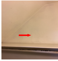
Office closet appears to have a crack on the wall recommend a qualified contractor to repair all that is necessary.
