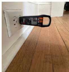
There is an electrical outlet that does not appear to be powered in the Upstairs Bedroom left of the master bedroom .
