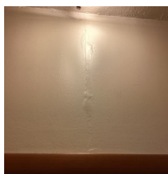
There is what appears to be a typical crack in an interior wall in the Closet between kitchen and living room.
