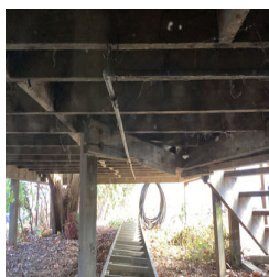
There are damaged materials on the steps for the Deck.
