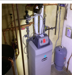
Boiler Heating System
