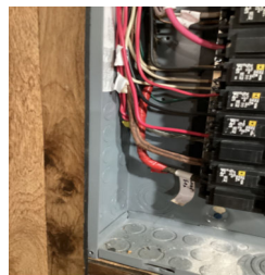
Main Electrical Panel Board Enclosure in the basement
