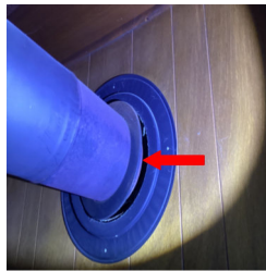
Fireplace in the Living Room, the finish piece around the exhaust pipe is out of place.
