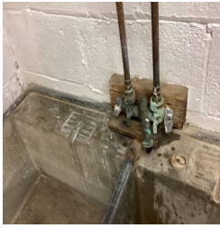
A sink fixture is loose in the Laundry Area.
