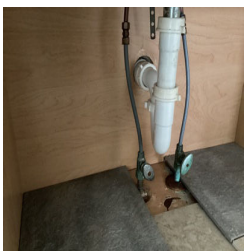
A sink water supply line is corroded in the Master Bathroom.
