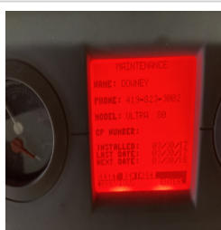
Boiler Heating System
