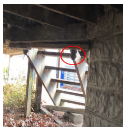
The steps are improperly supported on the Deck.
