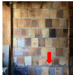
There is an area of noticeable repair to an interior wall in the Garage.
