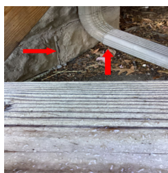
There are no splash blocks installed on some of the gutter downspouts for the roof drainage system for the Roof of the Home. Also in this picture there is cracking on the block foundation wall.
