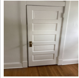
Office closet door doesn't shut properly
