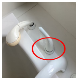
A tub hot faucet knob leaks in the Master Bathroom.
