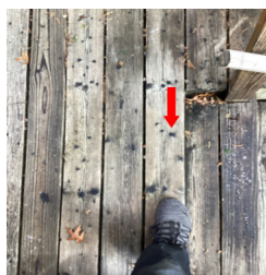
There is bounce in the Deck when it is walked on.
