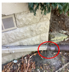
No splash block underneath the downspout.
