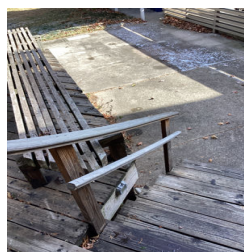
A baluster is missing on the Deck.
