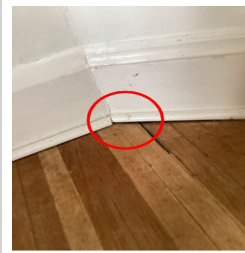
Upstairs Bedroom left of the master bedroom baseboard quarter round loose.
