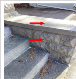
There is deteriorated mortar on the steps for the Front Porch.
