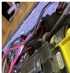
There is an open knockout in the Main Electrical Panel Board Enclosure in the.
